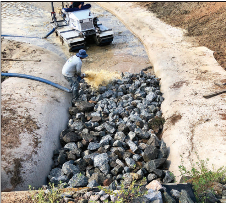
A combination of dredged sediment and excess fill from the project fills the SOX system and then secured by pound the staking system subsurface.
