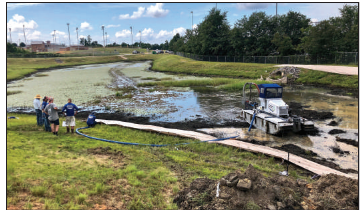
Using an amphibious work boat, pond sediment is dredged into the SOX system to stabilize the shoreline.
